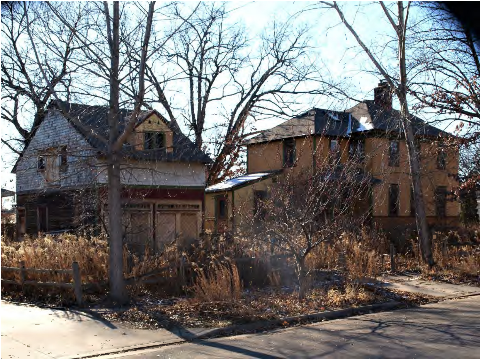
Dwight and Clara Watson House_000 barn and house on Delos tree viewed from northeast, east and north elevations, camera facing southwest
